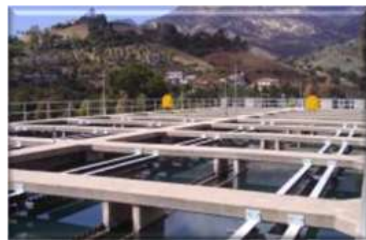
City of Santa Barbara Cater Treatment Plant
