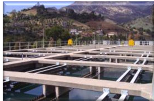
City of Santa Barbara Cater Treatment Plant
