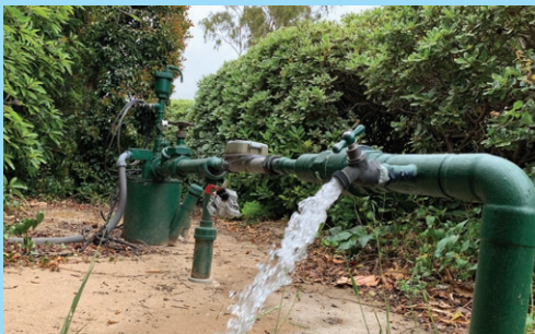
Groundwater wells, source from the Montecito Groundwater Basin.
