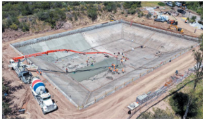
Construction is underway on Terminal Reservoir, the first of eight essential water storage facilities to be upgraded through the MWD's Reservoir Seismic Retrofit and Replacement Project (courtesy photo)
