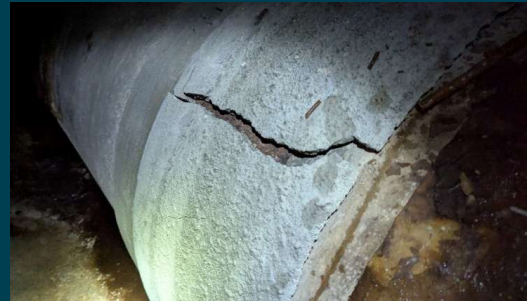
Type 4: Severe cracks 1/2" to 1"
