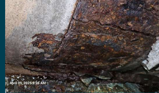
Type 6: No mortar, joint ring cracked/ compromised
