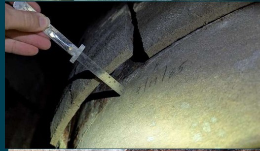
Type 5: Mortar separating from pipeline from exfoliation of joint ring
