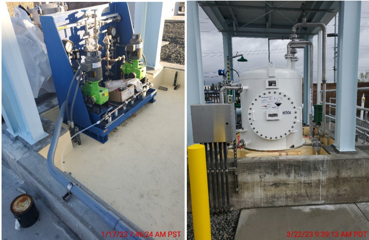
Figure 1 – Sulfuric Acid Chemical Feed Pump (left) and Dosing Tank (right)
