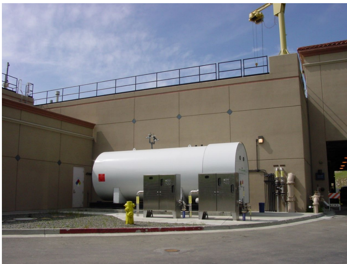
Figure 2 – Carbon Dioxide Storage Tank and Equipment Panels
