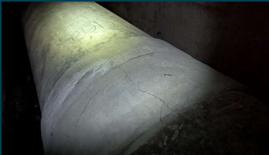
Type 2: Hairline cracks less than 1/8"
