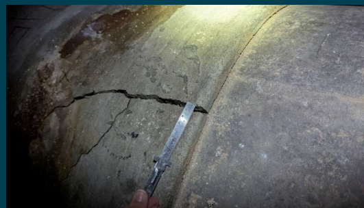
Type 3: Moderate cracks 1/8" to 1/2"
