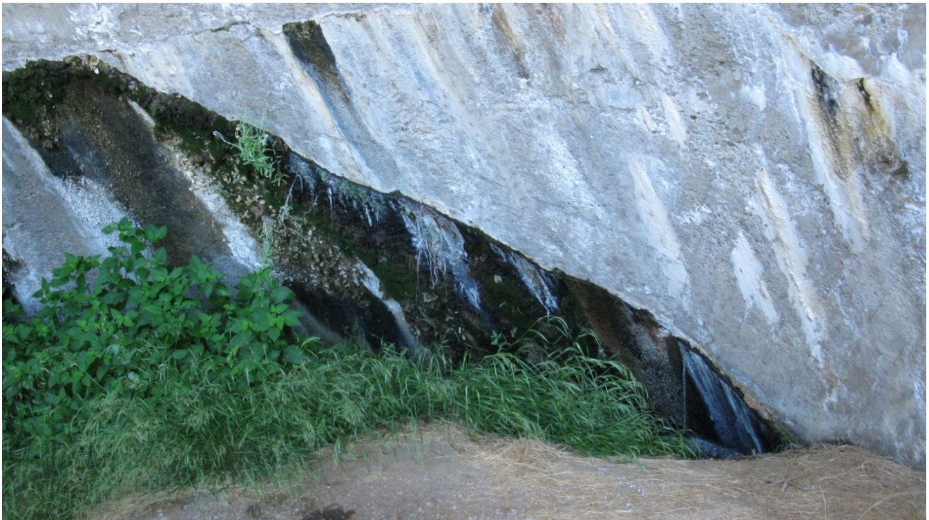
Seepage through lift joints in Bay 5 of the multiple arch section
